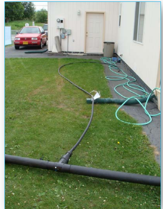
A temporary water line connected to a home through a hose bib.
