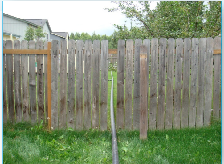
A photo of a temporary water service line extending from an on street fire hydrant through subdivision yards to neighborhood homes.
